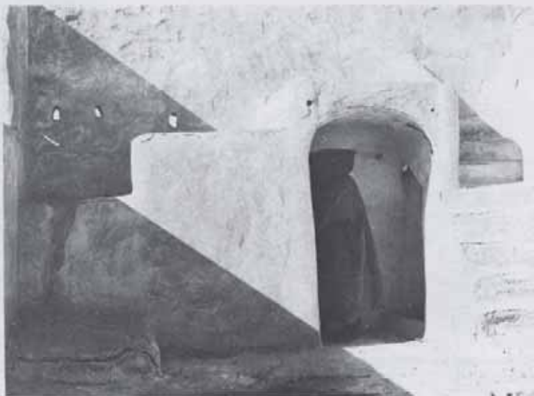
A roof terrace showing the stair exit and an opening over the courtyard below.
